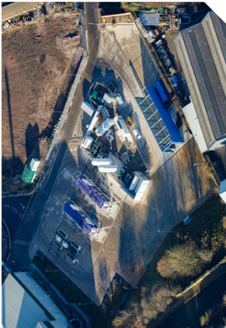
Image courtesy of Tyseley Energy Park
